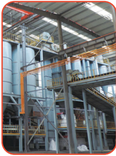
Clay Sand Production Line
