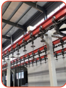
Paint Baking Line
